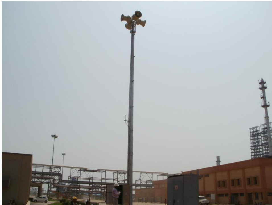
Technician working on a HPSS16 at the refinery
