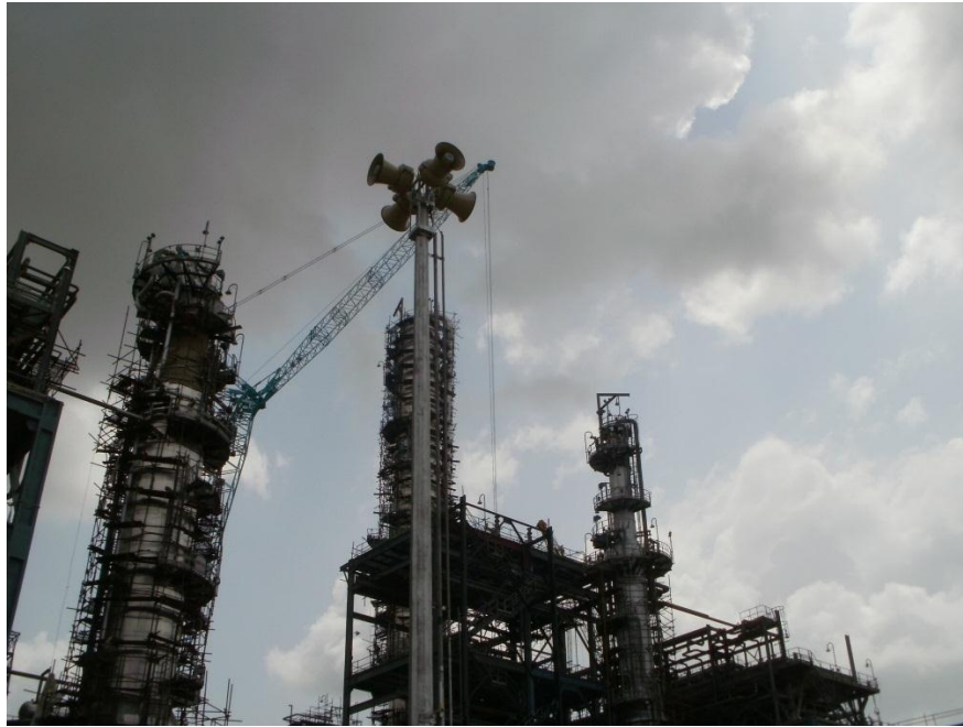
ATI Systems’ HPSS16 siren installed at the HMEL GGSR refinery
